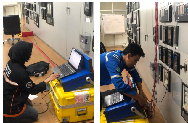
Fig. 3. Trial of protection relays
