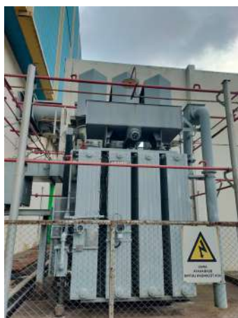
Fig. 1. Transformer (Source: PT PLN Nusantara Power UP Gresik)
