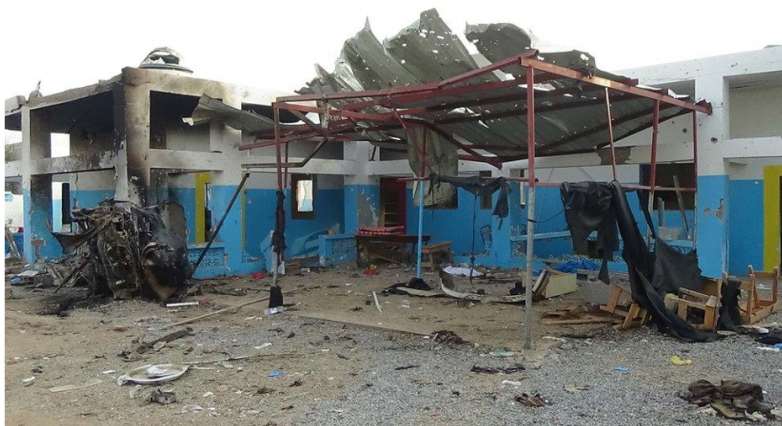
Fig. 2. The hospital in the northern town of Abs was badly damaged during the conflict [16]
