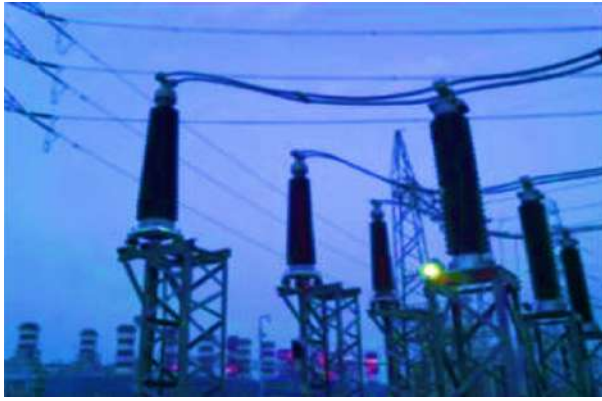
Fig. 2. The bushing being observed
